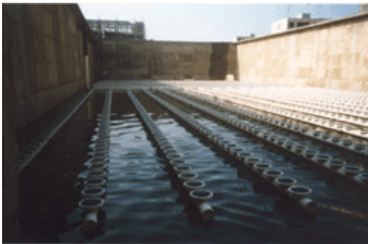
Fine bubble membrane diffusers
