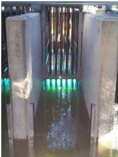
Horizontal UV system in a concrete channel
