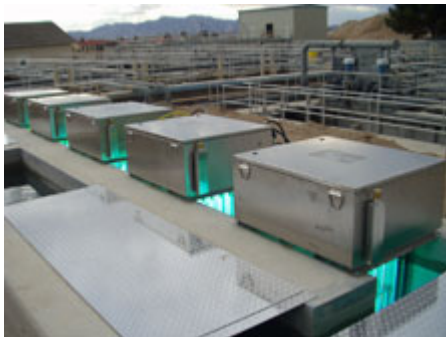
Vertical UV system in a concrete channel
