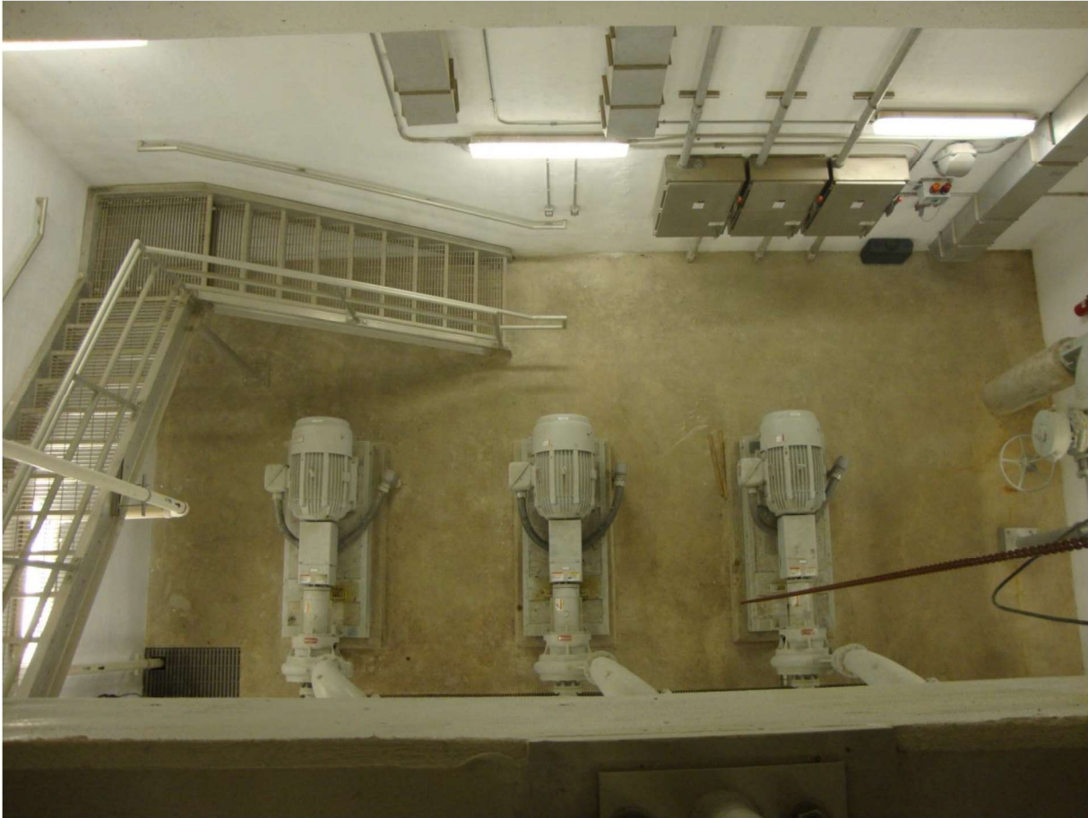
Figure 13 Gravity Lift Station Pumps
