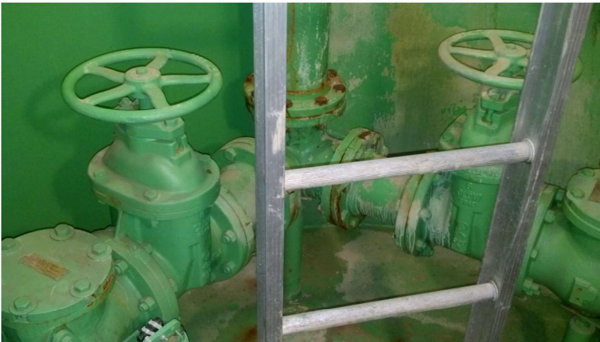
Figure 3 Rust and Paint Deterioration at the Stencil Lift Station
