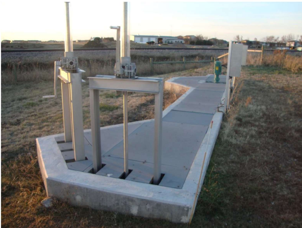
Figure 8 Inlet Channel with Grinder
