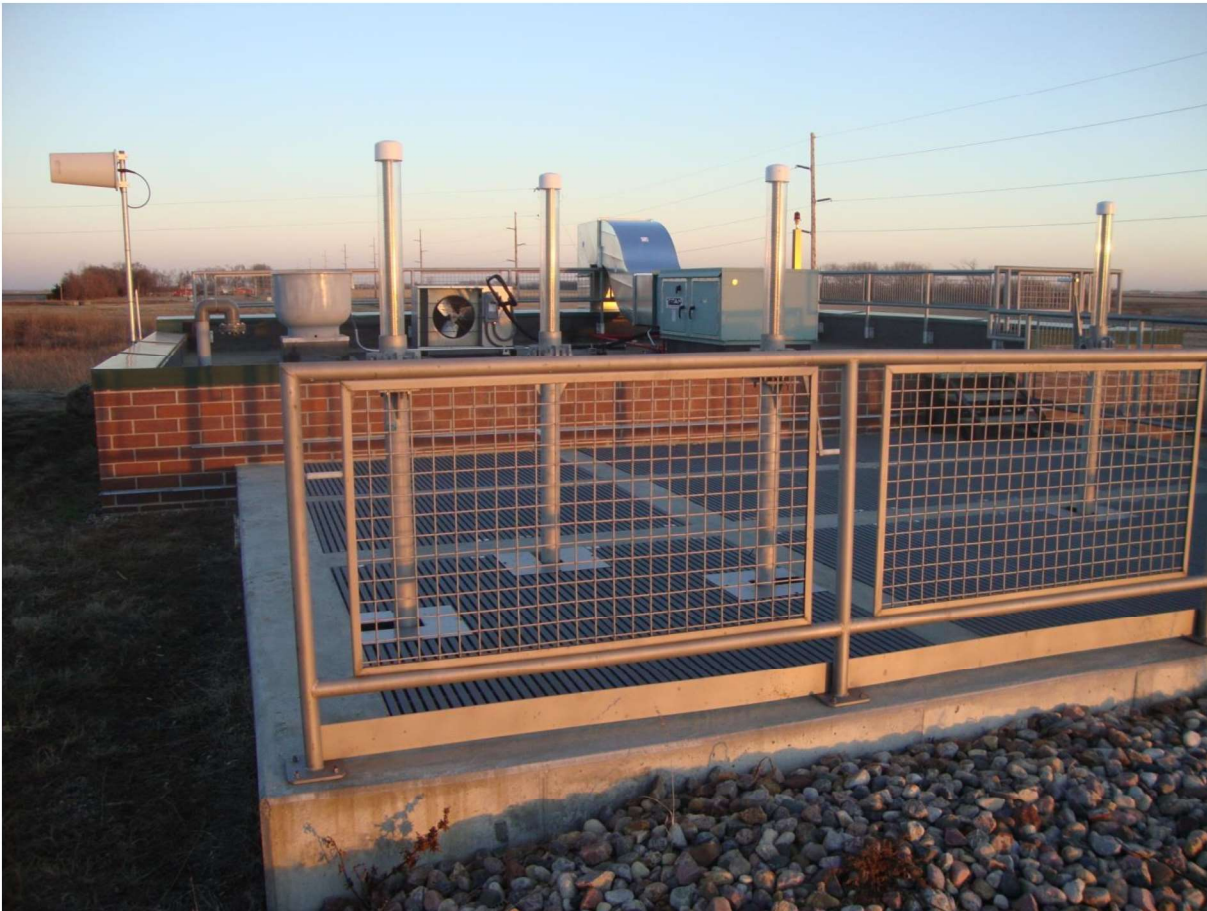
Figure 12 Gravity Lift Station
