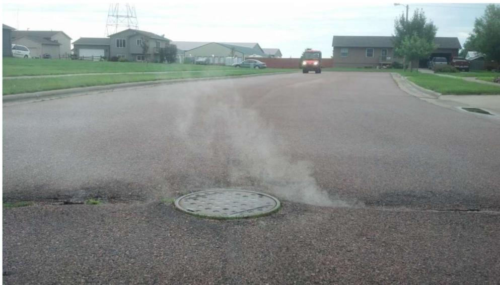
Figure 6 Smoke From Cracks Around Manhole
