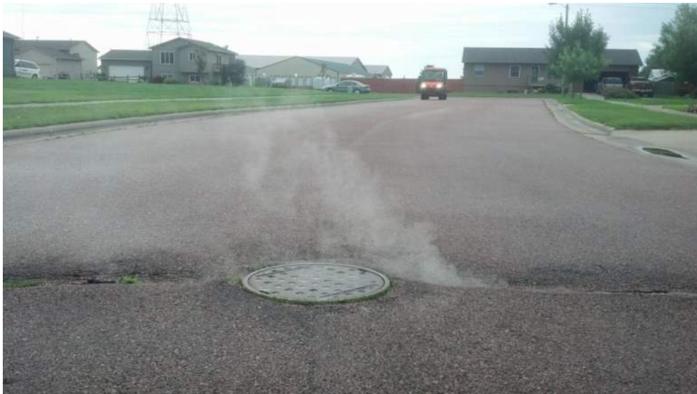
Figure 5 Smoke From Cracks Around Manhole
