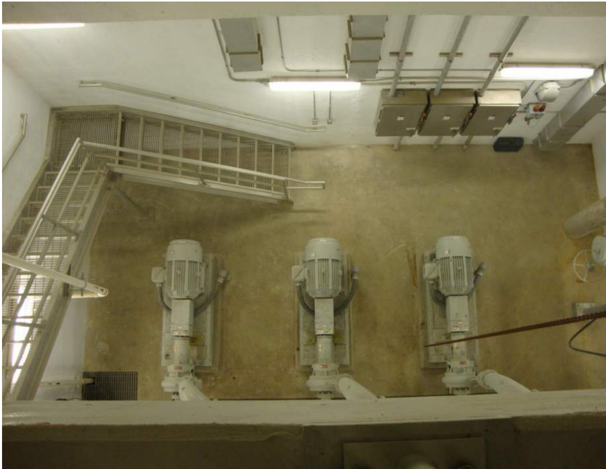
Figure 12 Gravity Lift Station Pumps
