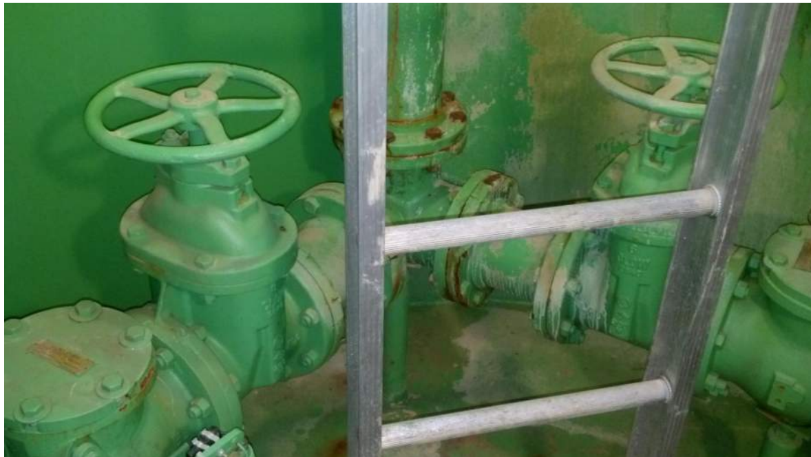
Figure 2 Rust and Paint Deterioration at the Stencil Lift Station
