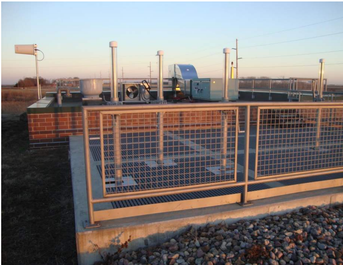
Figure 11 Gravity Lift Station
