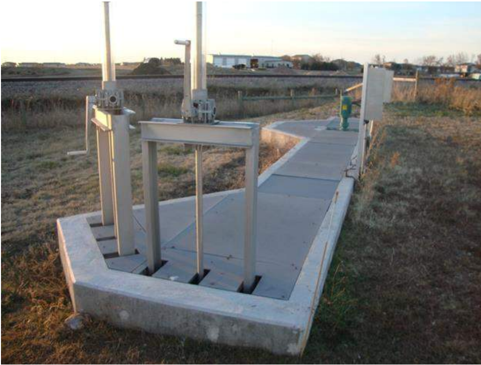
Figure 7 Inlet Channel with Grinder
