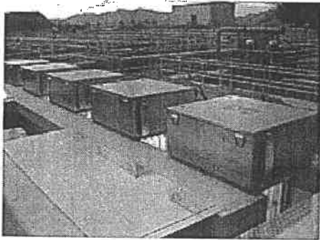
Vertical UV system in a concrete channel
